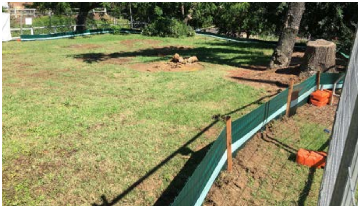
Figure 8. An appropriately installed sediment fence
