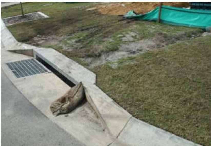
Figure 11. A sandbag kerb sediment trap collects sediment before it can enter the stormwater drain. Source: Catchments and Creeks Pty Ltd
