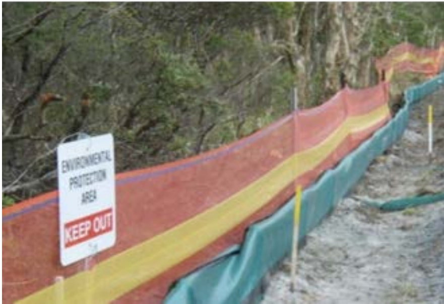
Figure 3. A example of a no-go area on a construction site, where access has been restricted to protect environmentally sensitive areas. Source: Department of Primary Industries and Regional Development – Fisheries
