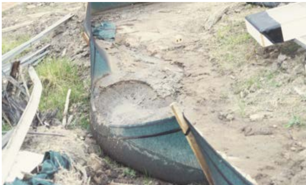
Figure 9. An inappropriately managed sediment fence. Source: Catchments and Creeks Pty Ltd
