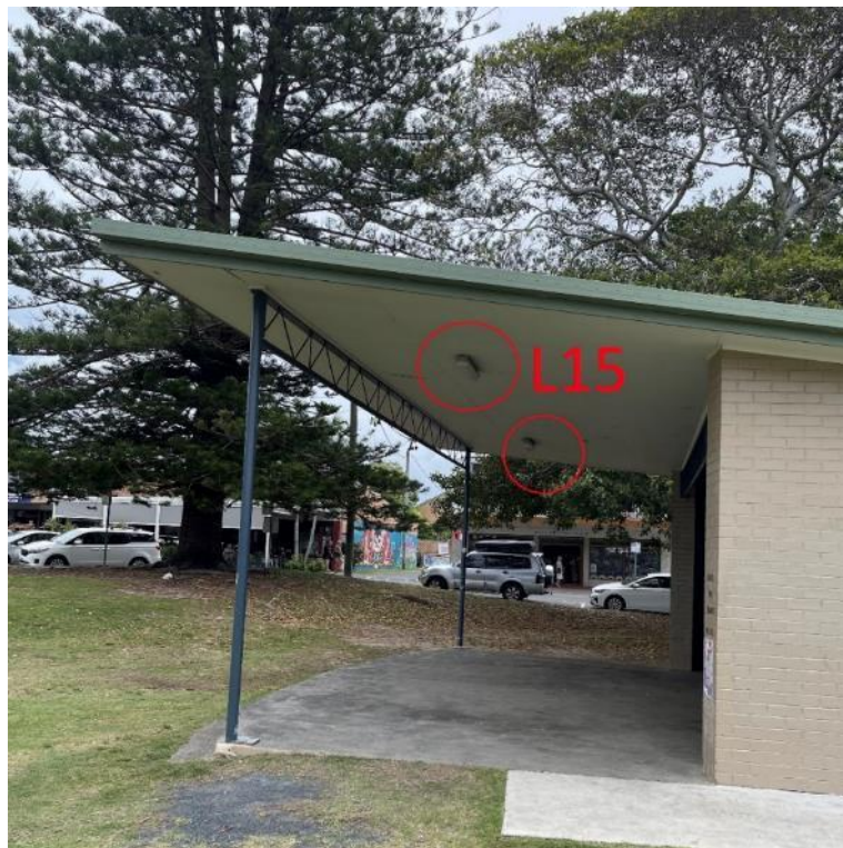
Plate 14: Terrace Park stage fluorescent lighting (L15) visible from Simpsons Creek.
