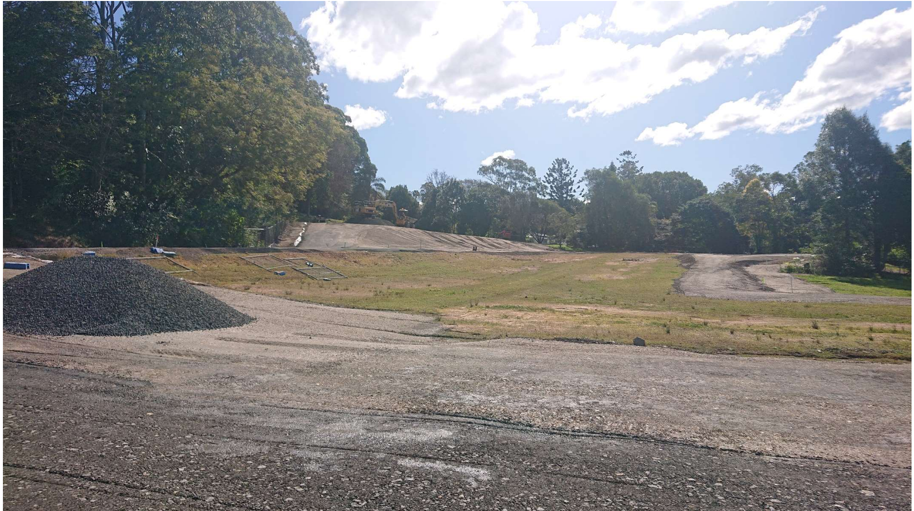
Plate B8. Northerly view of encapsulation area - overlooking Block A (grassy area) with Block C in top left and Block B in right (near tree) (16 th August 2022)
