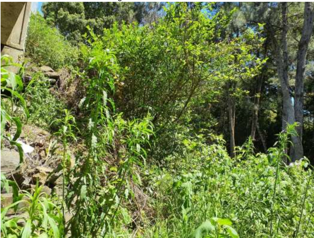
Plate C. View of vegetation below northwest bridge abutment requiring fill and scour protection.
